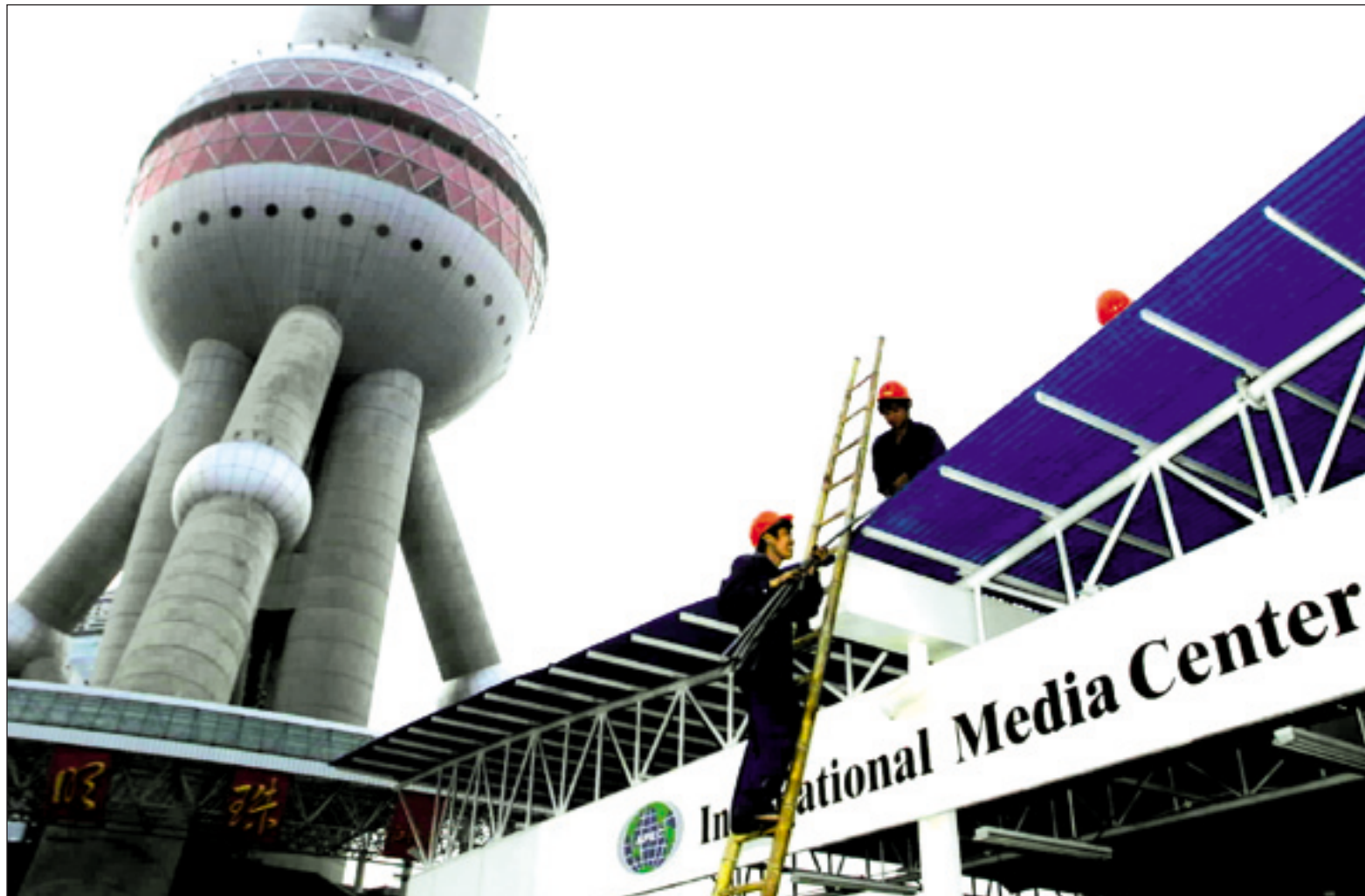
Workers put the finishing touches to the APEC Media Center under the Oriental Pearl TV Tower.
